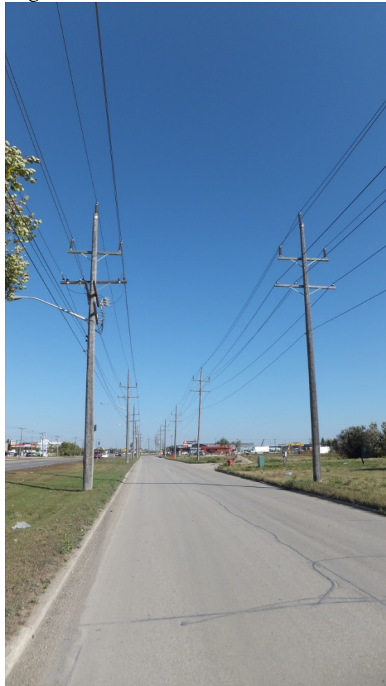
Figure 7: AC transmission feeder lines on both sides of a road
