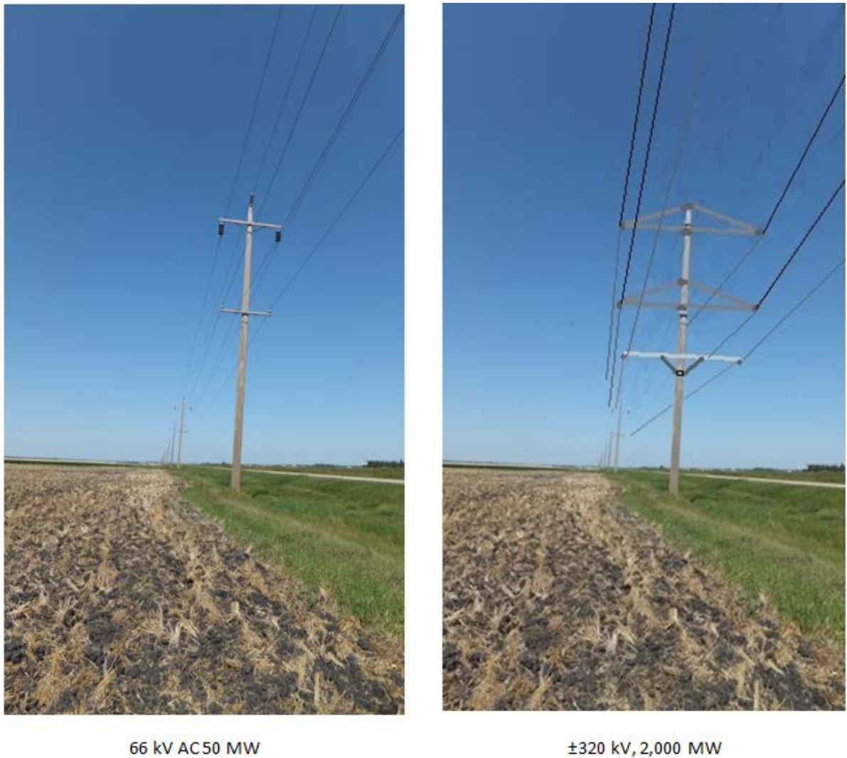
Figure 1: Compacted HVDC transmission with insulated cross arms compared with a conventional 66 kV AC roadside feeder. Note the shield wires beneath the active conductors for the HVDC transmission
