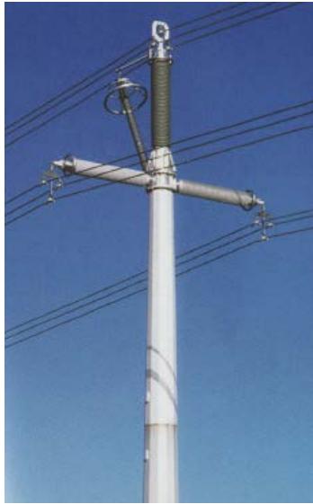
Figure 4: Insulated cross-arms for a compact 400 kV AC transmission tower (Courtesy of STRI)
